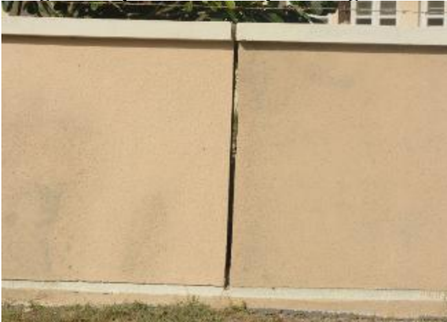
Gap between well plastered wall (Cl. A)
