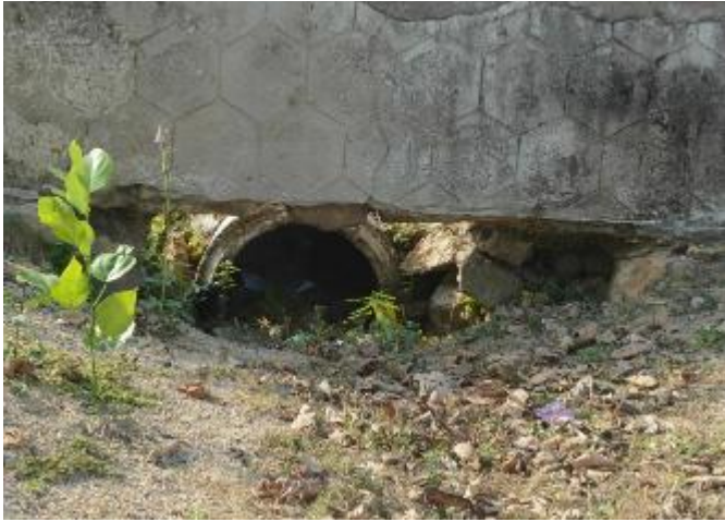
Unused culvert in front of school (Cl. A/D)
