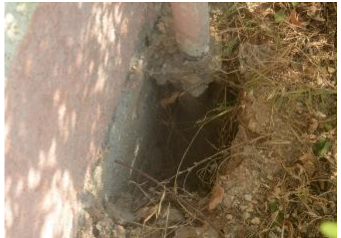
Cavity made with time in foundations (Cl. A)
