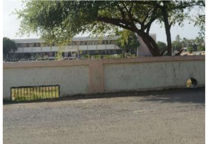
Metal net and hole in boundary wall (Cl. A)
