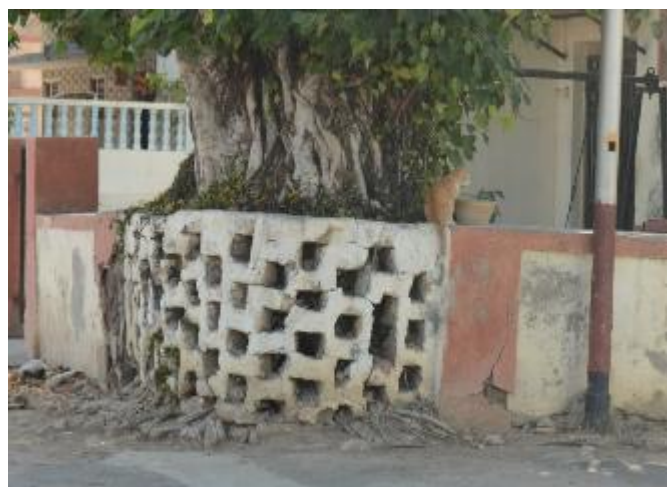
Tree guard/foundation with gaps (Cl. D)
