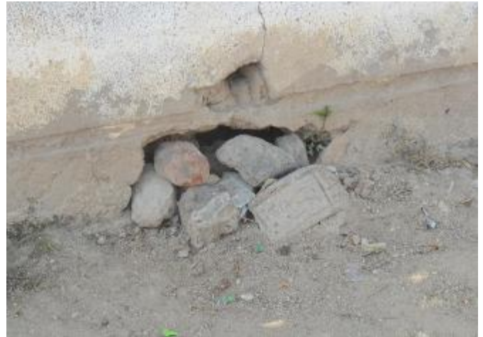
Poor filling of rocks in foundation cavity (Cl. C)
